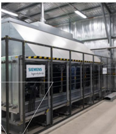
SIEMENS 1.25MW ELECTROLYSER
